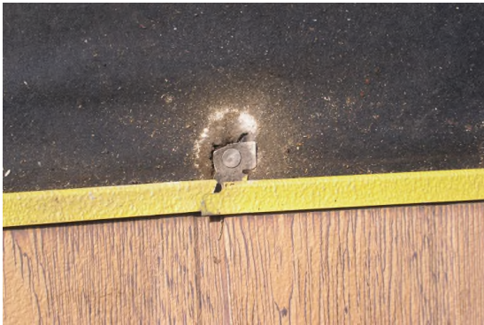
Example of a competitor product where the corner joint let in water and the nailing tab cut through the underlayment
